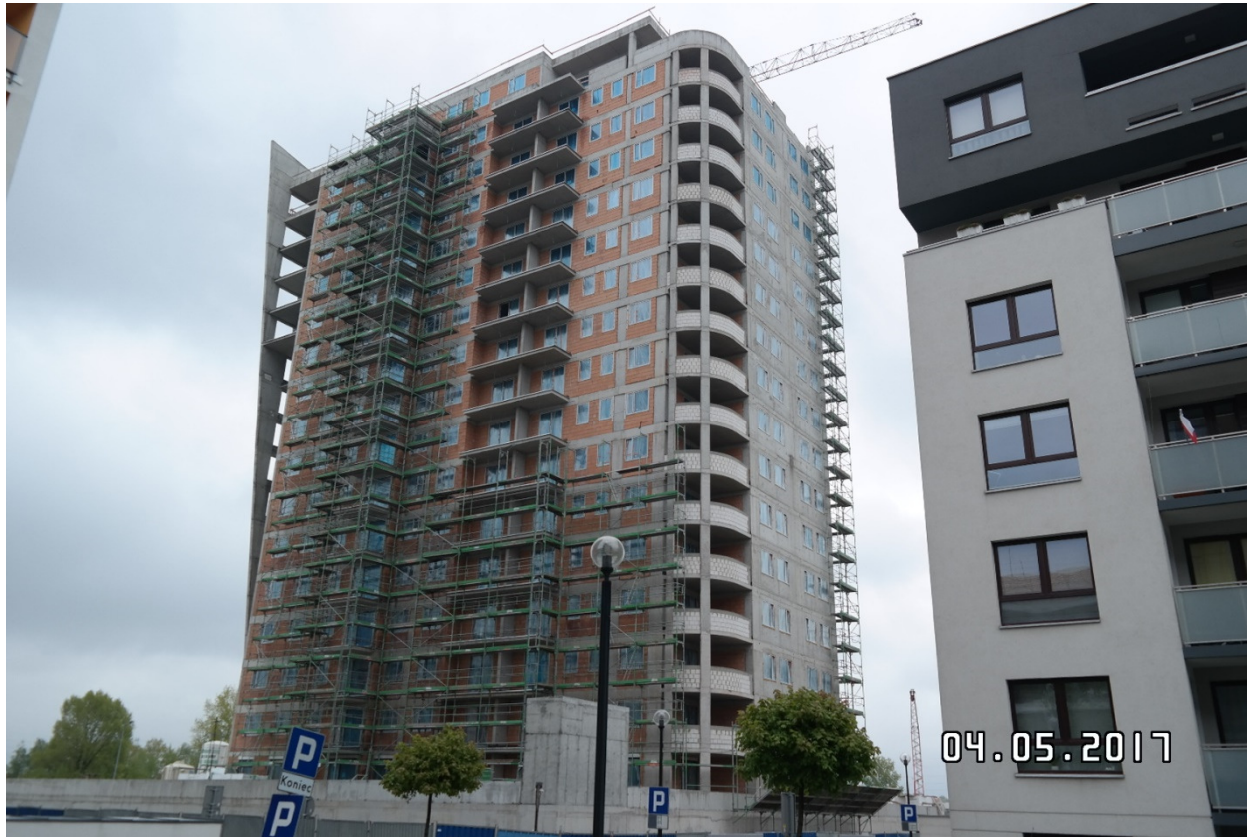
View of construction works in building 6.3, Apartamenty Innova, Wrocław (on the center of the image), On the right, stage IV (building 3.2) of Osiedle-Innova (Wrocław).
